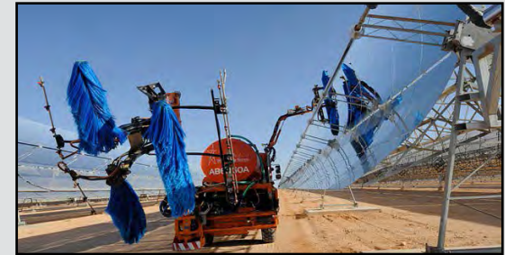
Morocco's CSP facility will be one of the world's largest.
